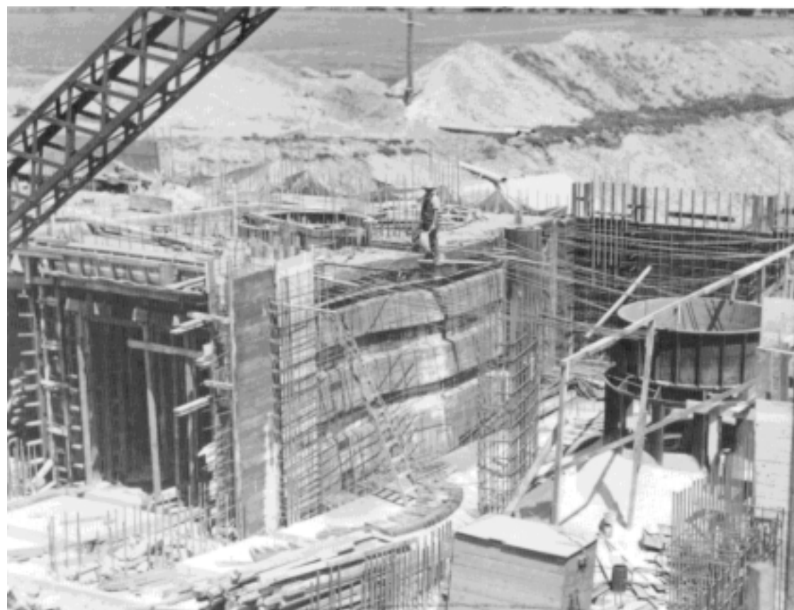
Standing atop the skeleton of the Monroe Powerhouse under construction, 17-year old Ralph Schmidt hoses down cement, keeping it wet. The cement had to stay damp for 11 days.
