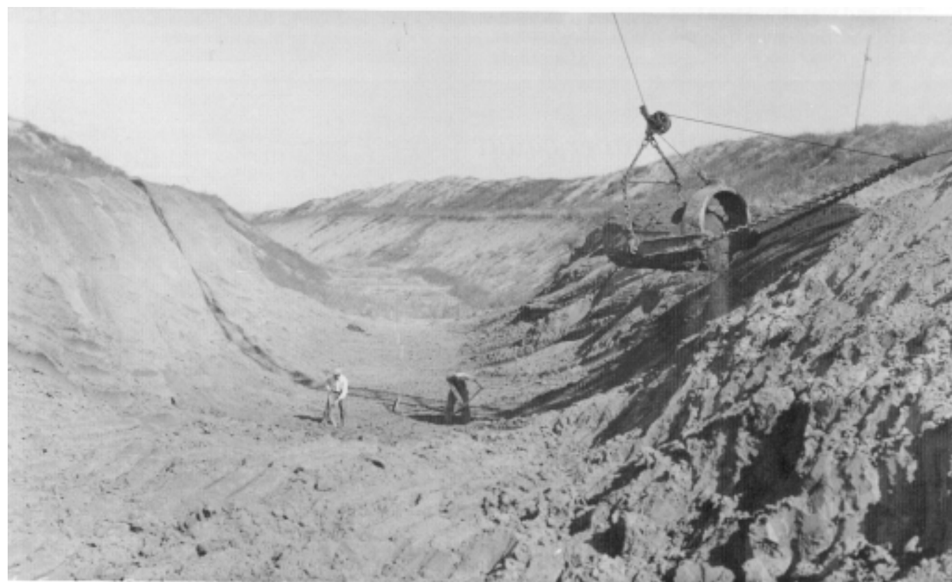
A dry ditch, a very large dry ditch: the Loup power canal under excavation in 1935.
